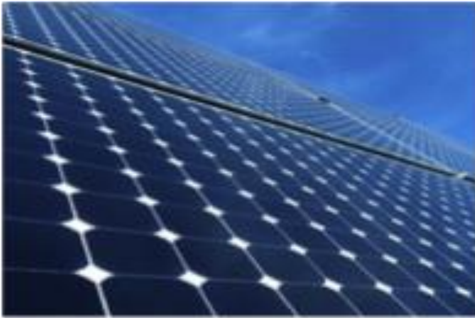
12 KWp PV Grid Connected solar power plant
