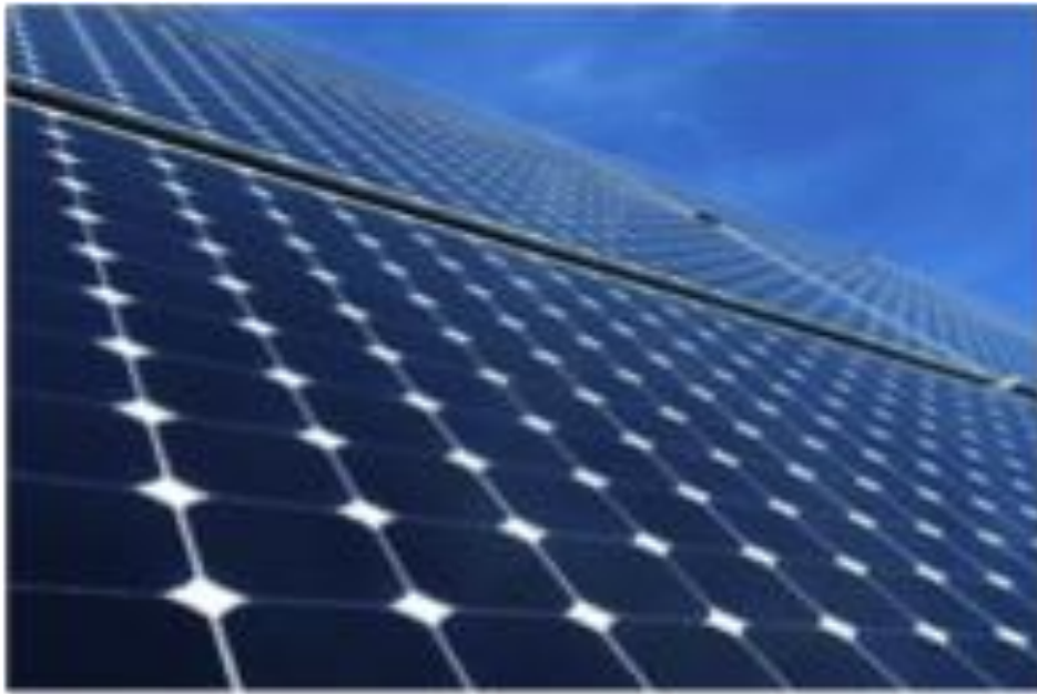
12 KWp PV Grid Connected solar power plant
